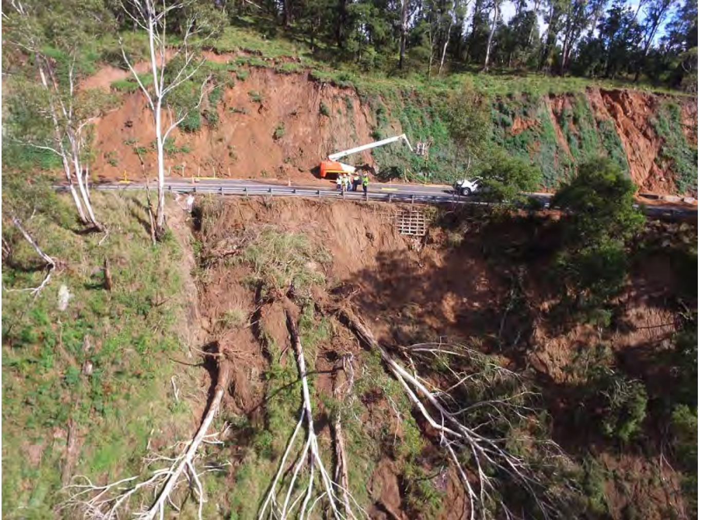
Figure 5 Landslip at Jenolan Caves Road, Hampton 10
